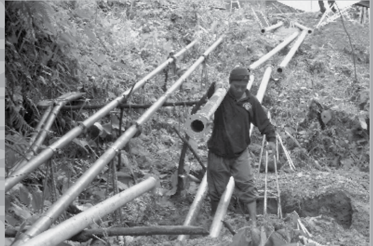
Photo by Michel Maupoux, Steel Pipes for Tres Hermanos Ram Pump System , near Bacolod, Negros Occidental, Philippines, June 2010.
